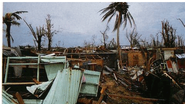
Damage on the island of Guadeloupe after Hurricane Hugo, 1989.
