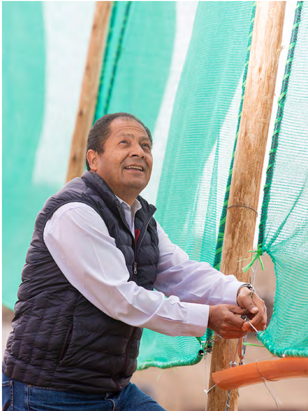
Ashoka Fellow Abel Cruz installs a net to harvest water from Peru's coastal fog.
